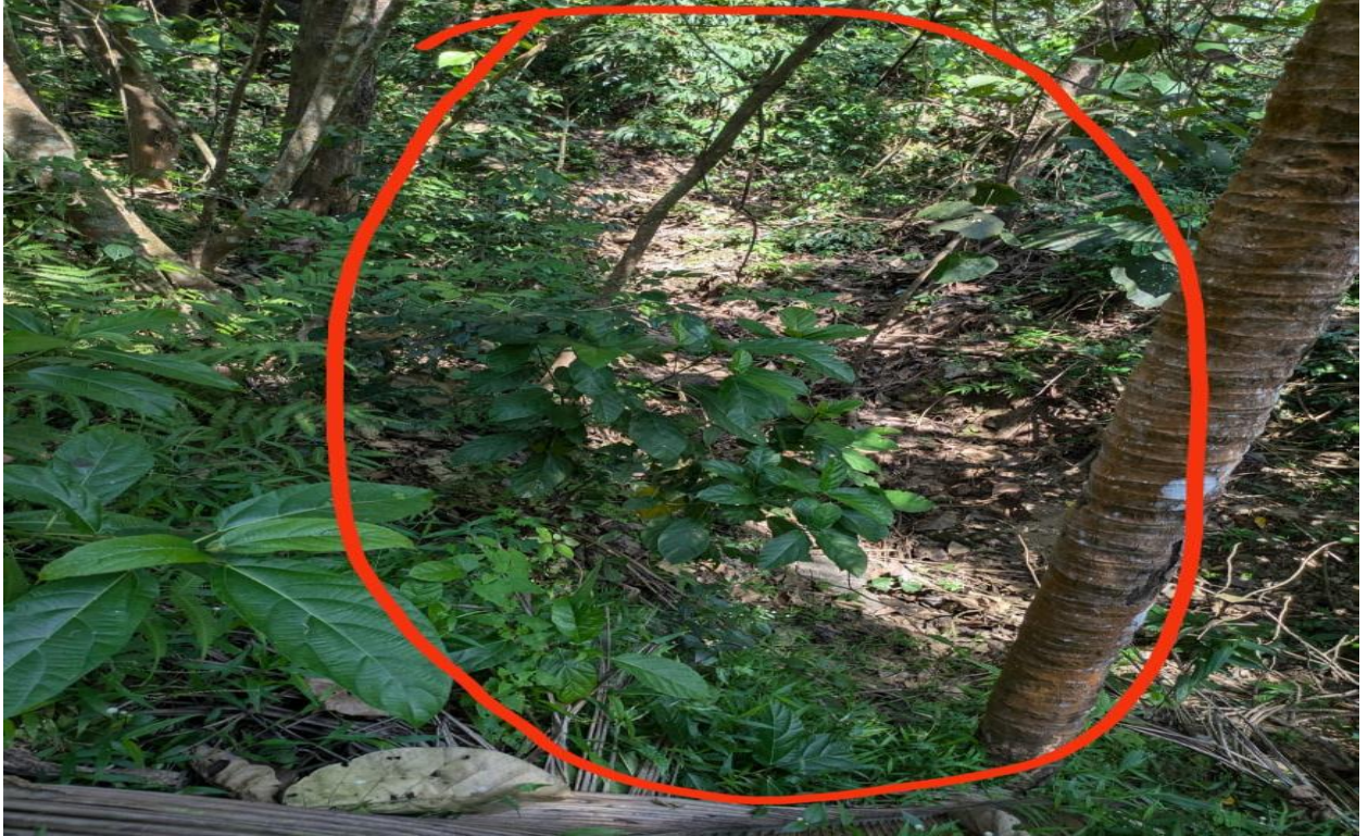
A landslide picture nearby the forest and quarrying area.
